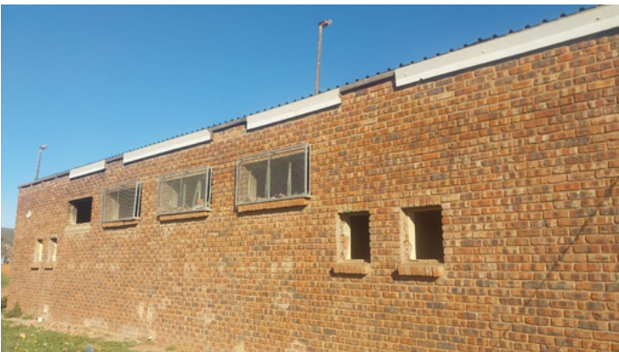
Windows removed and roof vandalised.
