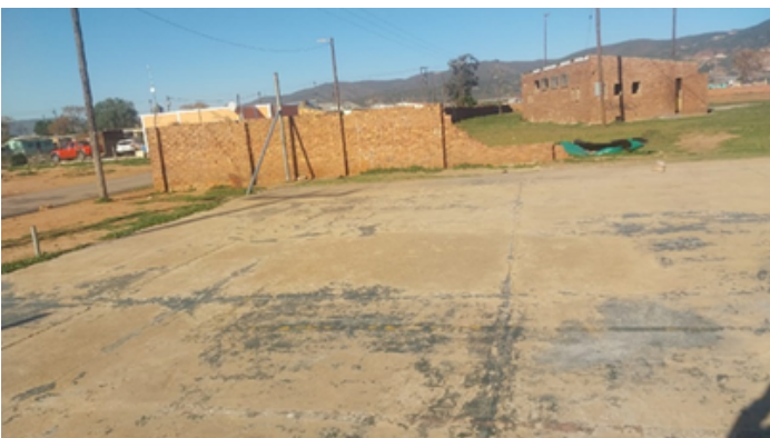
Boundary wall broken down.
