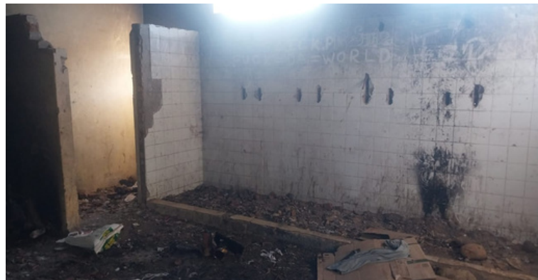
Changing rooms completely vandalised.
